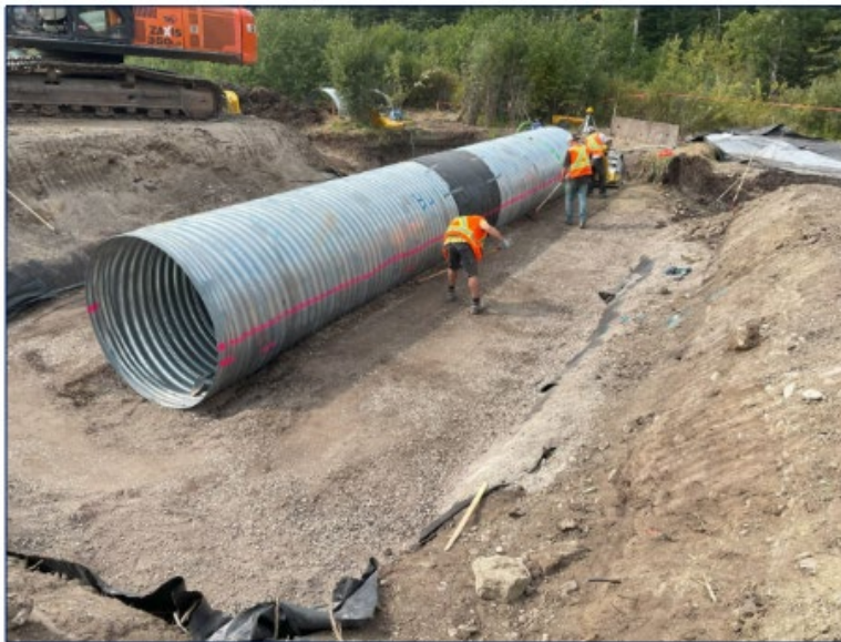
September 9, 2024 Clay seal and gravel backfill completed to 25%. Culvert was marked with 150 mm lifts and required testing marks.
